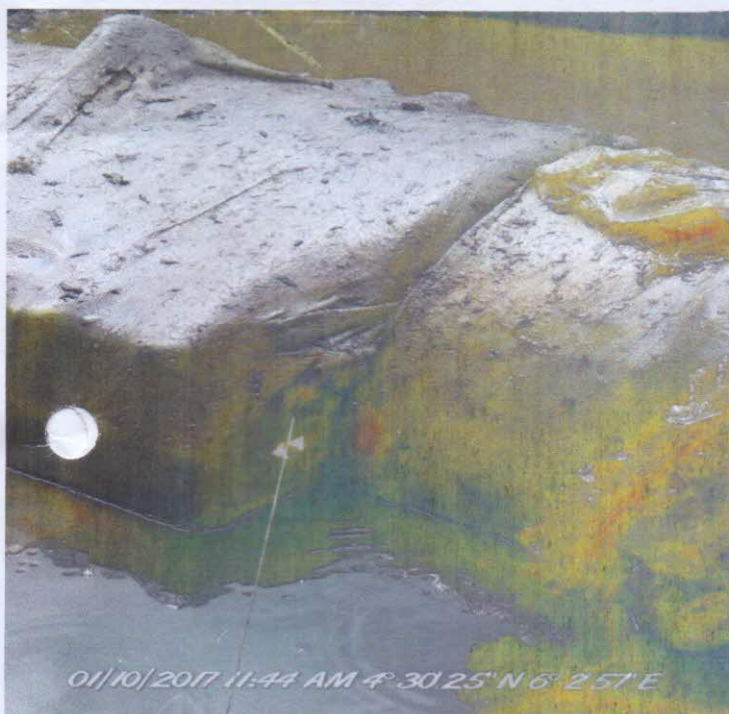
Figure 2 SOURCE OF THE LEAKAGE FROM THE FAILED CLAMP (2) AFTER EXCAVATION.
